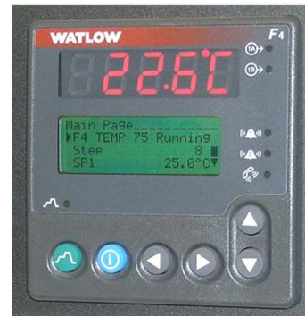
Figure 9 Watlow F4 Temperature Controller
