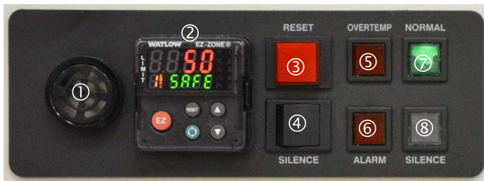
Figure 16 Tempgard IV Controller
